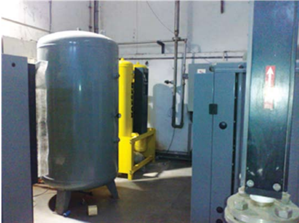
Fig. 2.3.1 New drier system incorporated in the existing Stirling plant
