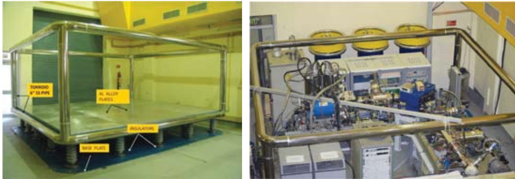
Fig. 2.2.1 (left) View of the 200 kV high voltage platform; (right) view of the 18 GHz HTS ECR ion source and beam transport components installed on the platform.
